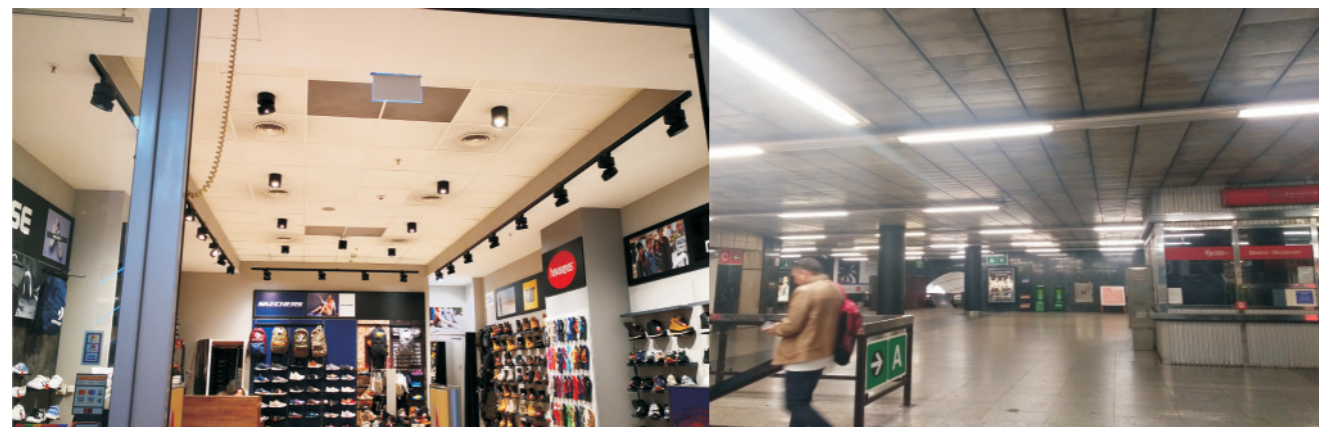
Application : Class II light fixture
